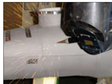
Recreating cooling holes in the same position and with the same specification as the original
